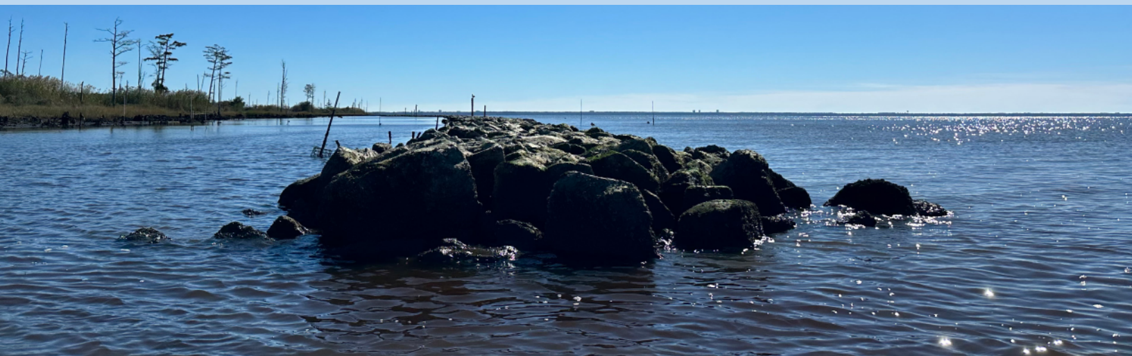
Rubble mound breakwater at the Swift Tract living shoreline project (extreme low tide) in Mobile Bay, Alabama. Photo credit: Bret Webb
